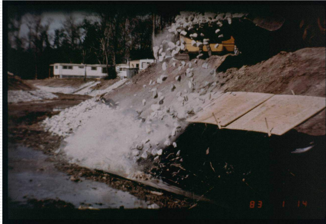
Excessive Drop Height / Damage
