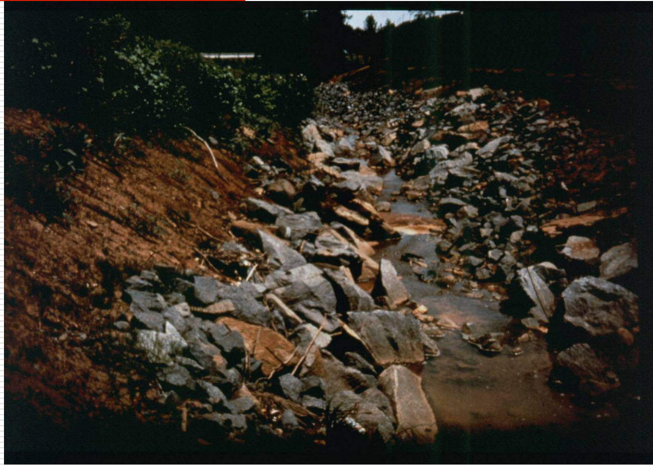
An Undermined Hard Armor System
