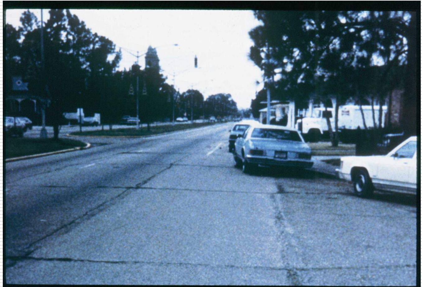
Typical Cracked Pavement
