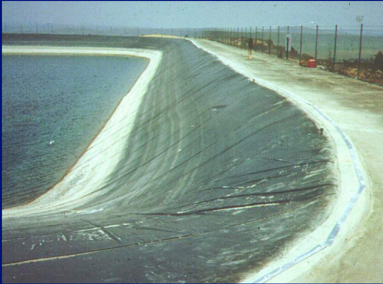
(Lined Potable Water Reservoir)
