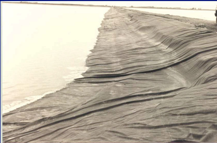
(Pond With Failed Subgrade)
