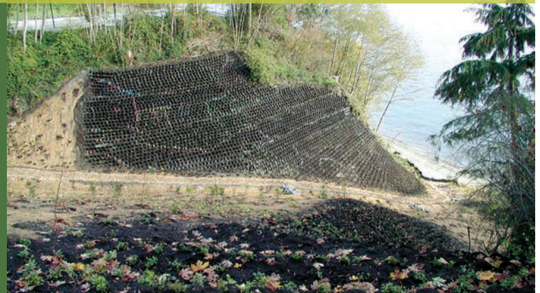
Top Left: Ravine erosion, note sediment trap at ravine mouth Top Right: Geocell placement on steep slope with confined work area Bottom: Completed 30m-high geocell slope
