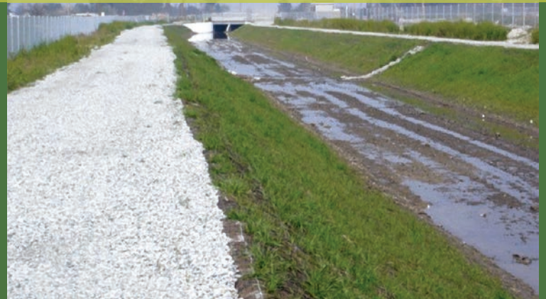
Top Left: Channel during TRM installation—Note protected and unprotected slope conditions. Top Right: More rain—Note rock in place failure, with intact TRM. .
