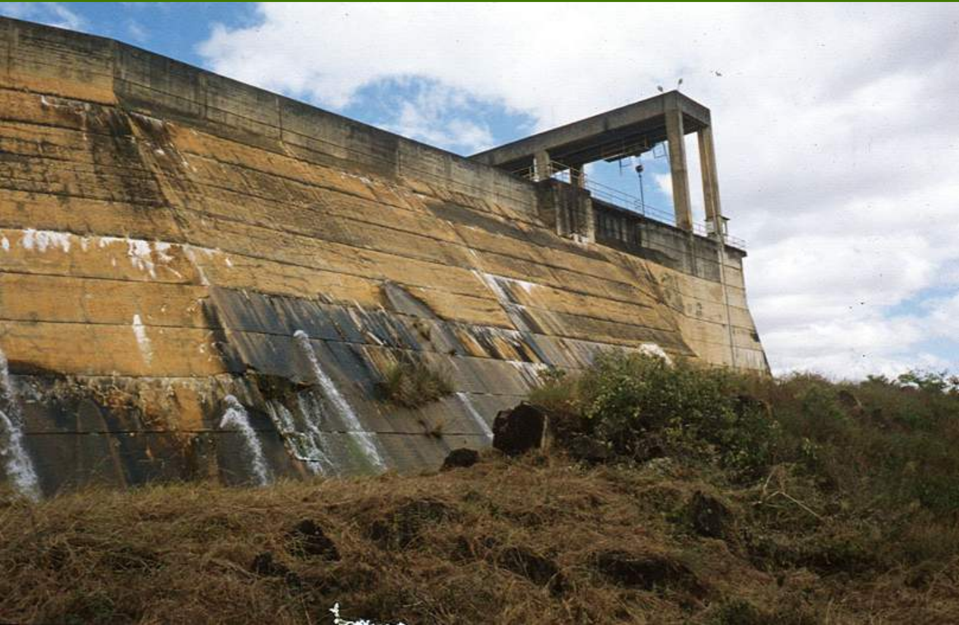
Downstream Seepage in Concrete Dam
