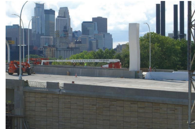
Geogrids provided reinforcement in the bridge abutment of the new Interstate 35W bridge that replaced the bridge that collapsed in catastrophic fashion on Aug. 1, 2007. This photo shows the final stage of construction including the finished retaining wall, the bridge deck, and the downtown Minneapolis skyline.
