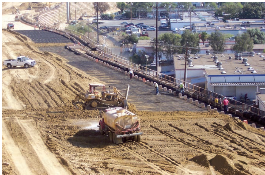
Geogrids provided reinforcement allowing engineers to build this massive retaining wall, within a limited footprint, in this Interstate 5/805 project in San Diego County, California.
